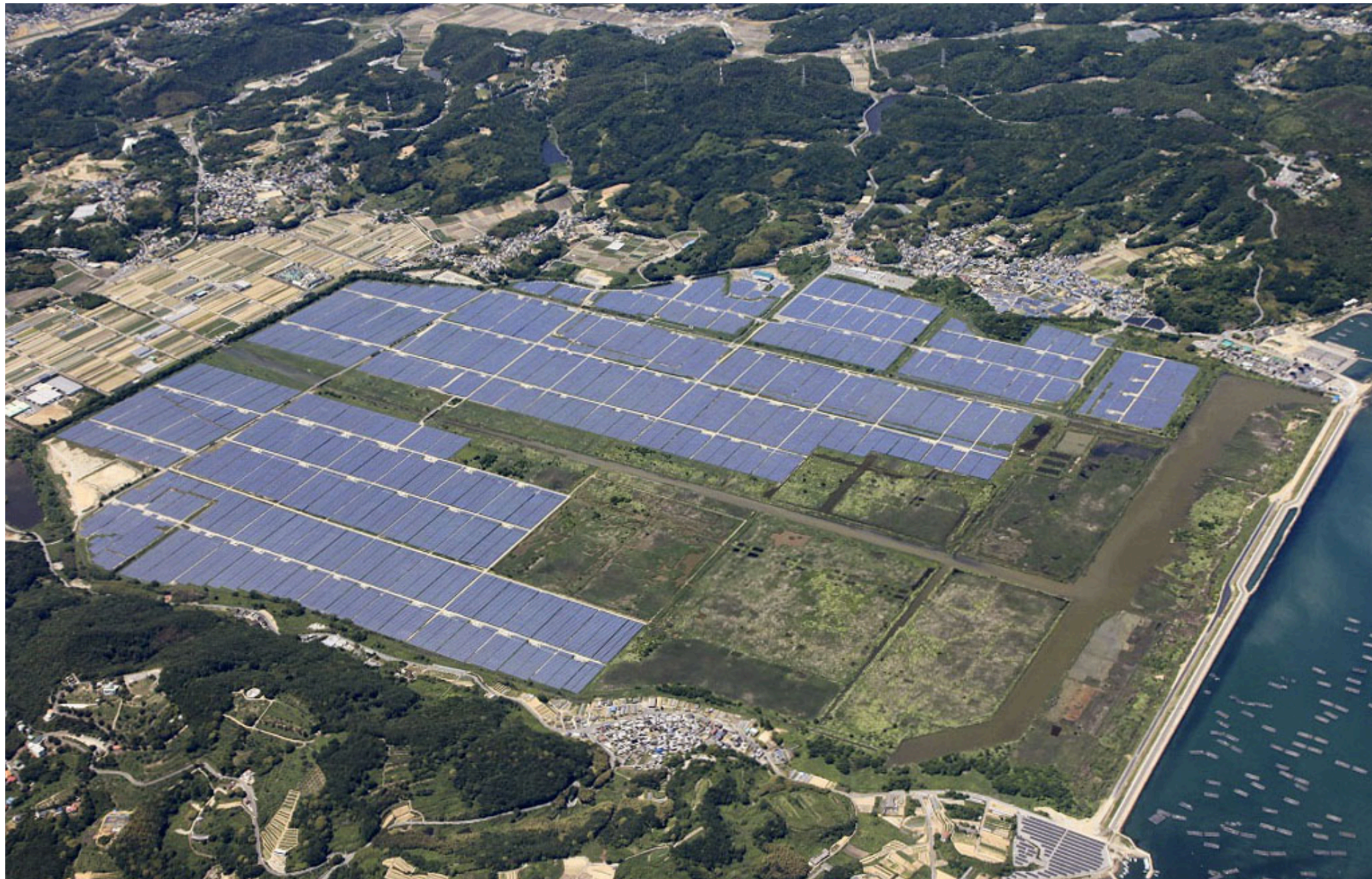
Setouchi Kirei Solar Power Plant
